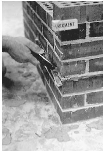
Figure 15-30 Trim flexible flashing flush with outside face of wall. (Photo courtesy BIA.)
